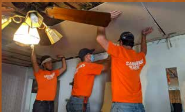
Jayme Baker (center) works alongside a team of other volunteers to remove sheetrock that was damaged from the storm.
